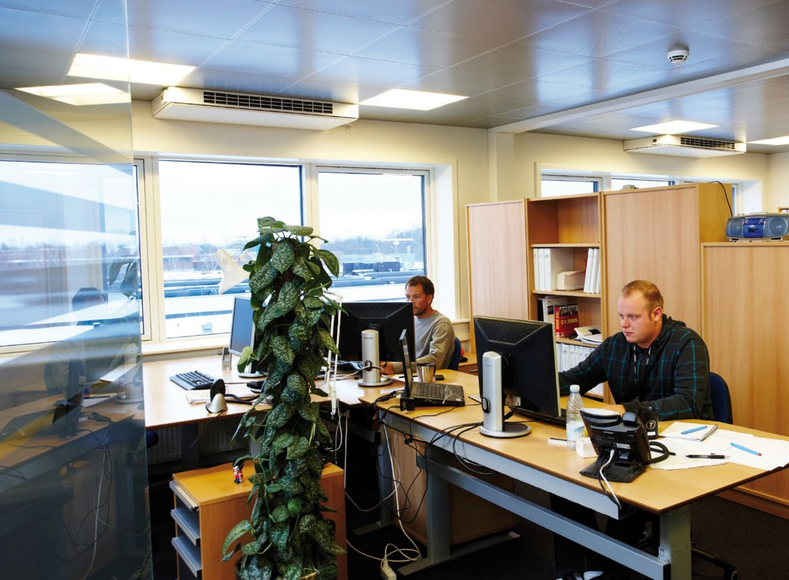
Two AM 300 air handling units are installed in the office, integrated into the ceiling.
